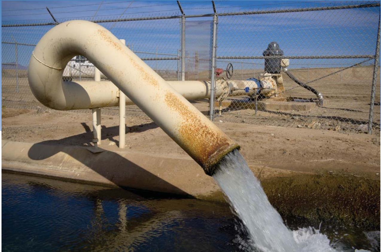
Typical groundwater well located in Yuma, Arizona. Photo credit: Andy Pernick, courtesy of the U.S. Bureau of Reclamation.
