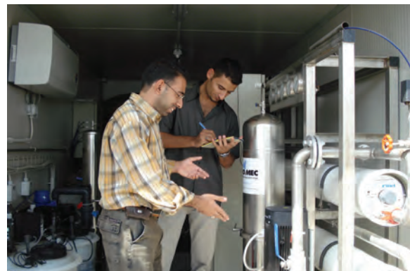
Figure 5 Water treatment equipment installations
