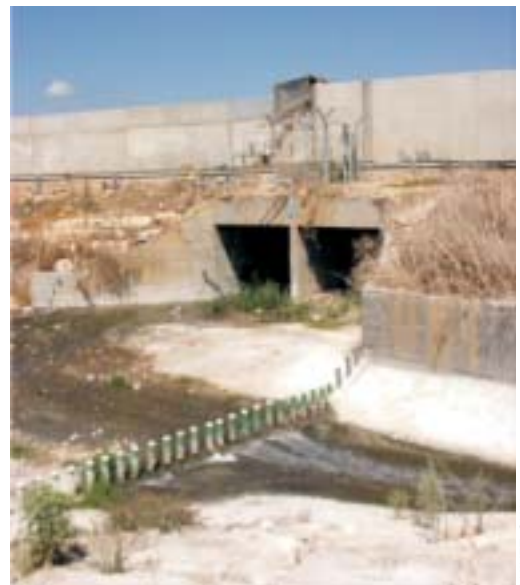
Untreated wastewater from Tulkarm is deviated into an Israeli emergency treatment plant to prevent pollution to the Alexander River downstream.
