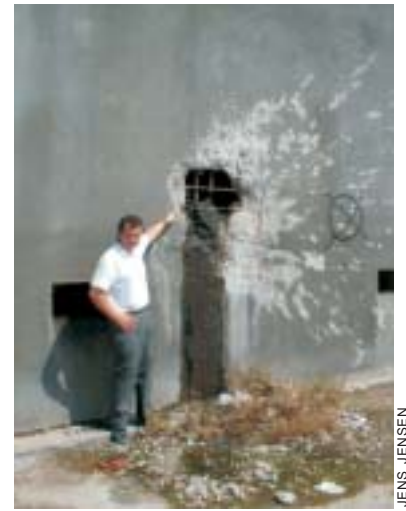
Damage sustained to the wastewater treatment plant in Gaza from Israeli military action
