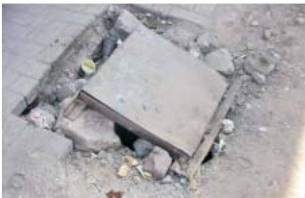
Sewage cover damaged by tank in the Jenin city centre
