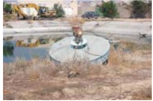
Broken aerator at Jenin wastewater treatment plant: spare parts are difficult to obtain
