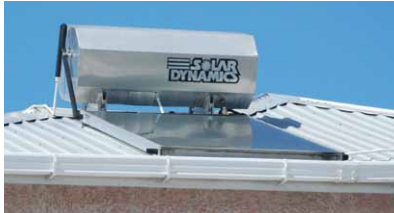
A Barbados solar water heater system – manufacturer, Solar Dynamics.
