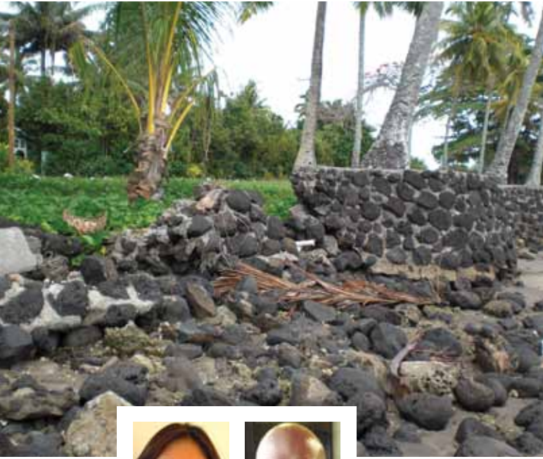
Figure 1: Independent Samoa: coastal defences are vulnerable to damage.
