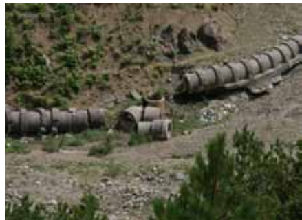
Failed water diversion channel
