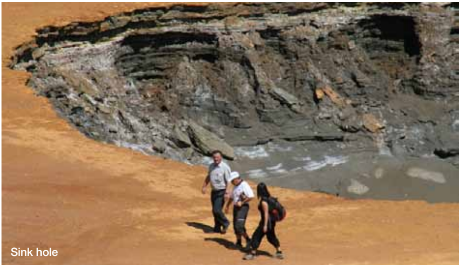
Top view on Rreshen tailings dam, second sinkhole outside the picture on the right
