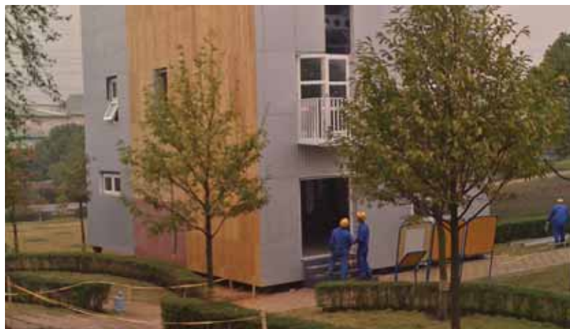
A Broad Air sustainable building can be established in just three days
