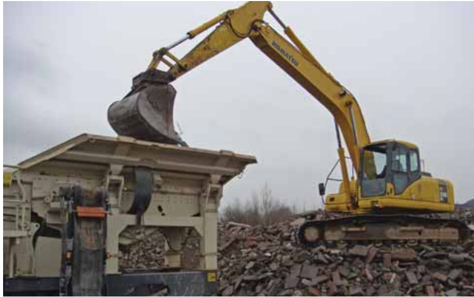
Piles of debris could be seen at Leigu township in Sichuan Province, which was devastated by the earthquake
