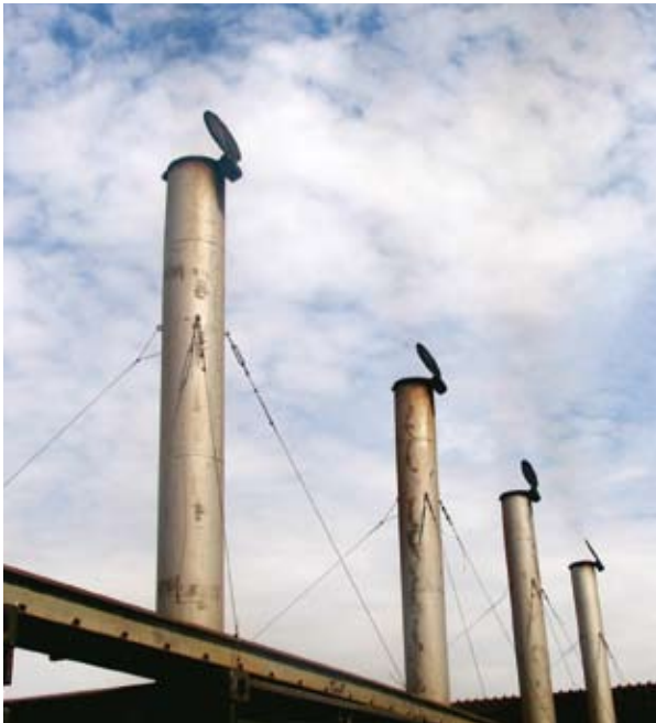
Diesel generators rented by the Government of Rwanda to compensate the electricity shortage
