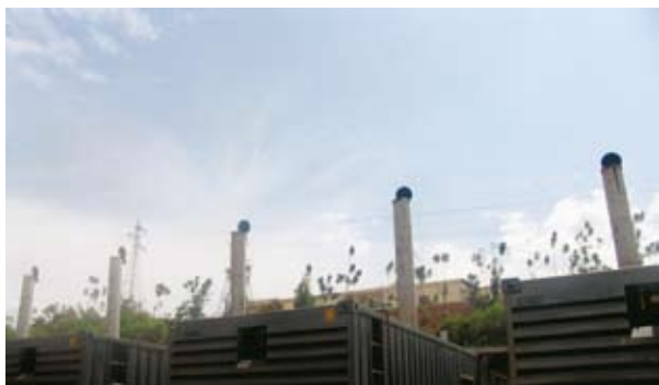
Diesel generators in Gikondo - Kigali City
