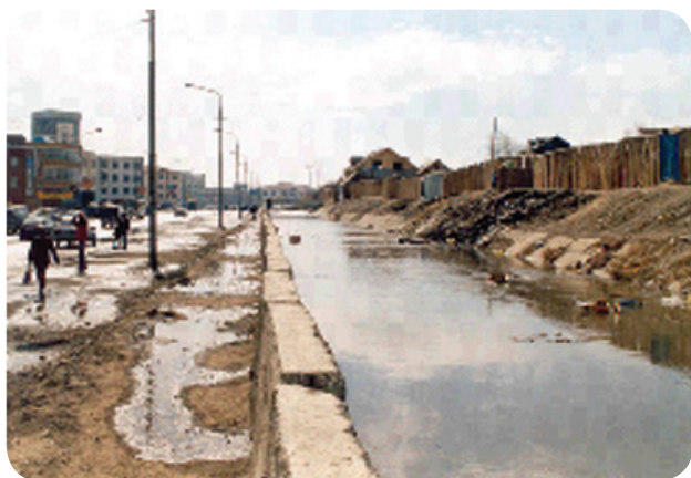
Figure 19. Flood protection channel functioning during rain in Ulaanbaatar (Source: Davaasuren, 2009)
