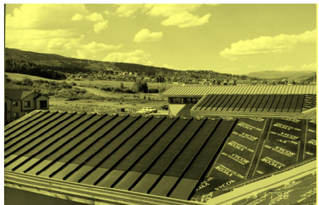
Solar cells have been directly installed as part of this building's roof (courtesy NREL).
