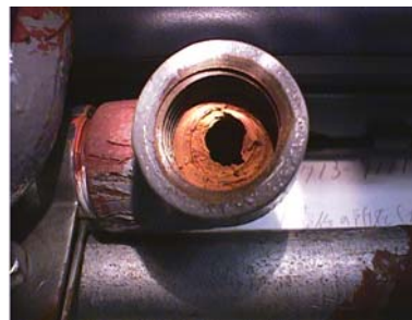
Figure 17: Blockage of pipe joint
