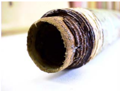
Figure 16: Corrosion of pipe joint
