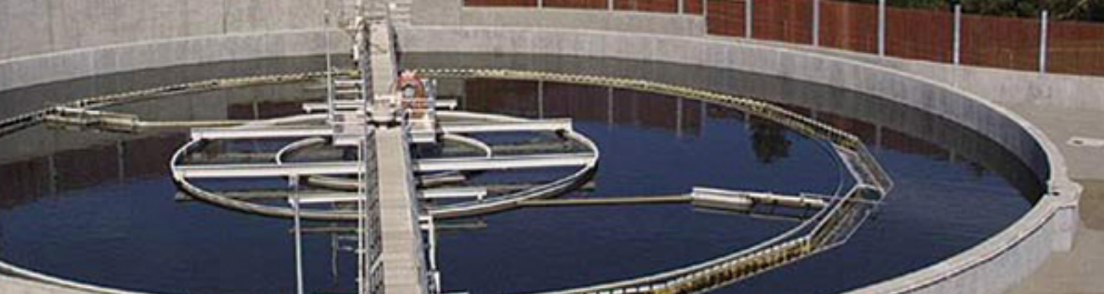
Wastewater treatment center
