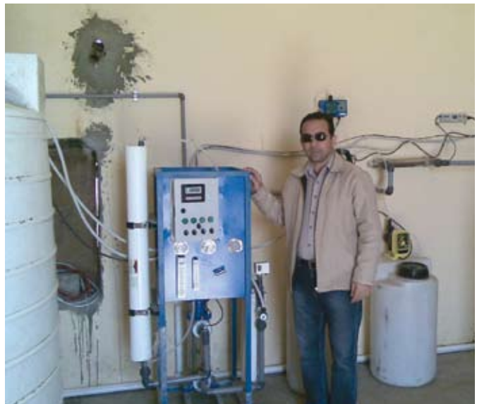
Desalination facilities supplied by the project Source: Mohamed Tawfic
