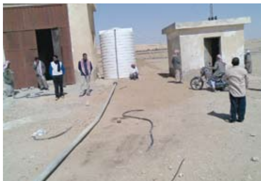
Installing water desalination unit at El Maghara, one of the community services the assessment project is providing
