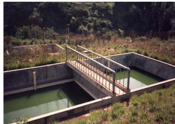
Static feed trickling filter with inexpensive volcanic rock media. Wastewater is dispersed via inexpensive perforated PVC pipe.
