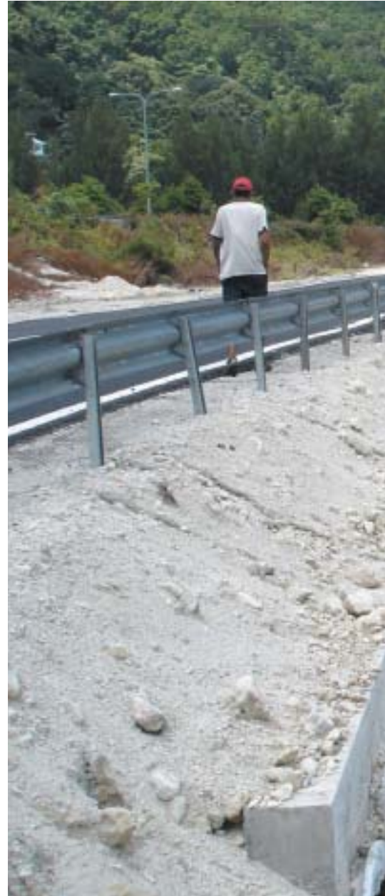
A reconstructed bridge on the airport highway following the tsunami. Credit: M. Collins
