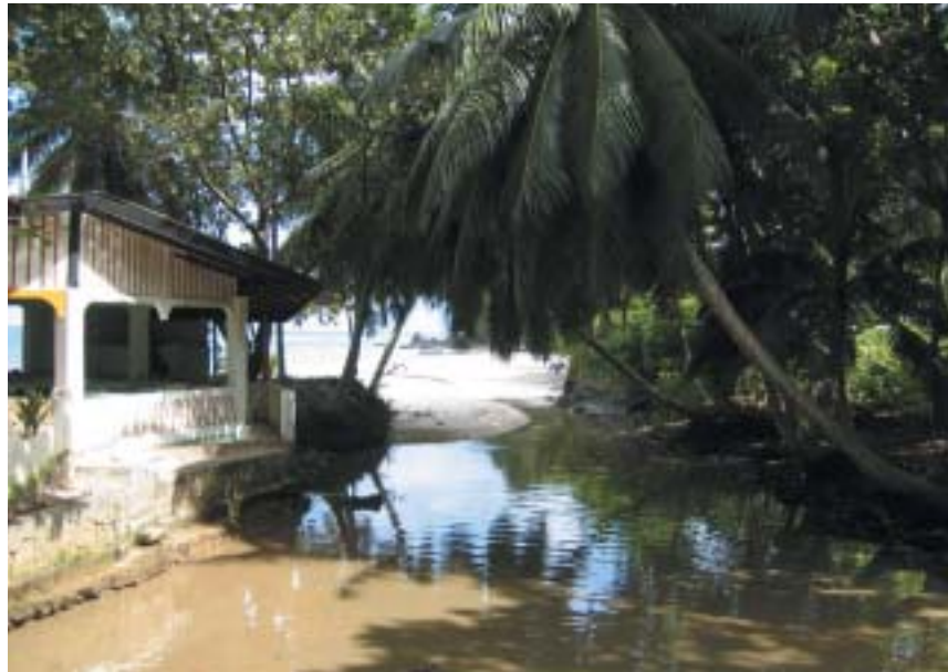
A clogged beach-side discharge channel. Credit: M. de Vries
