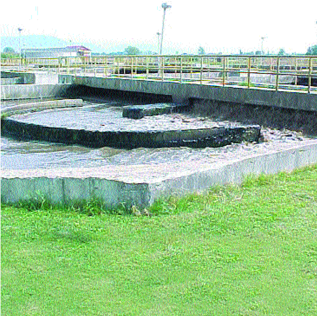
Struga treatment plant, Ohrid
