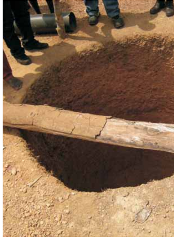
Drinking water well in the process of being completed in the Eastern province. Only half of Sierra Leoneans have access to an improved water source
