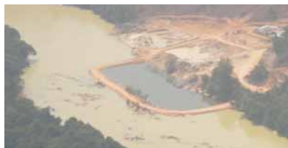
Artisanal diamond mining site in the heart of the mining region of eastern Sierra Leone. During the conflict, sites like this one were used by RUF rebels to extract diamonds for financing, resulting in pollution of major waterways and degraded land
