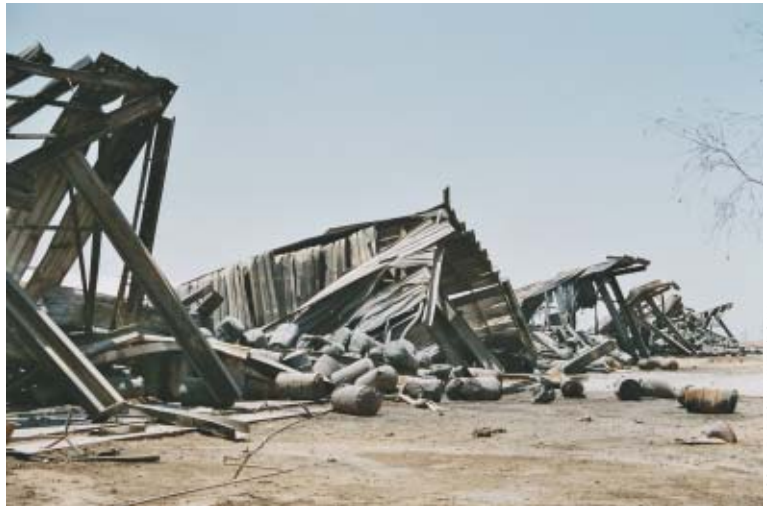
Midland storage facility prior to the outbreak of conflict (top left) Warehouses, containing highly hazardous chemicals, were completely destroyed by looting and arson
