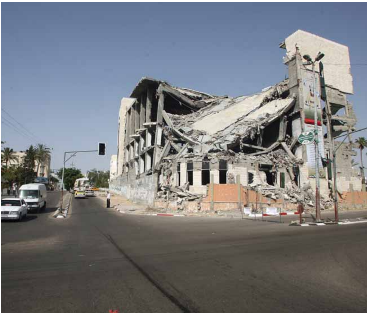
Hanging rubble in partially demolished buildings, like this one in Gaza City, poses a major challenge
