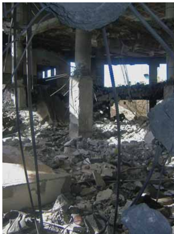
Damaged building in the Gaza Strip
