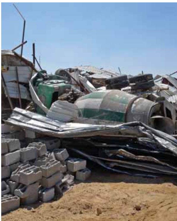
Bulldozed cement plant near Rafah
