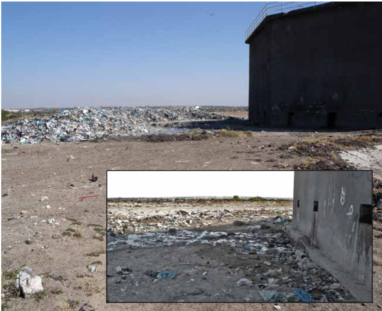
Leakage from the Az Zaitoun wastewater treatment plant trickling towers onto an adjacent pile of waste
