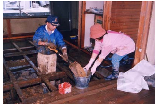
Residents remove silt from their homes
