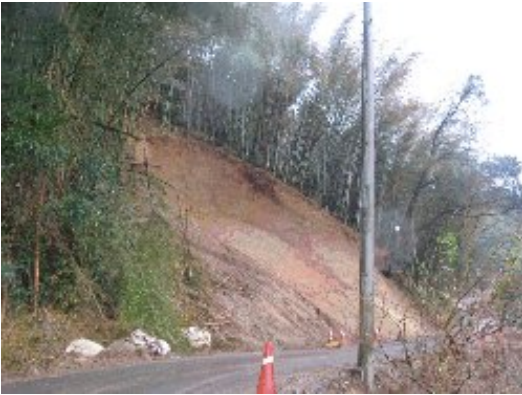
Poor forest cover and landslides
