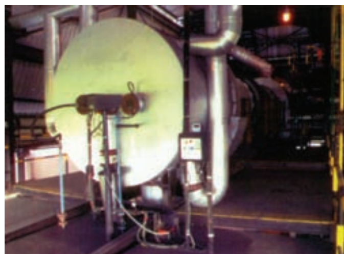
Rotary kiln furnace of the common hazardous waste incinerator
