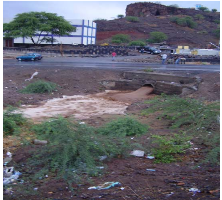
Hydraulic structures carrying stormwater at the roundabout between the airport road and the port road.
