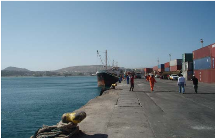
Result of scour action at the structure toe
