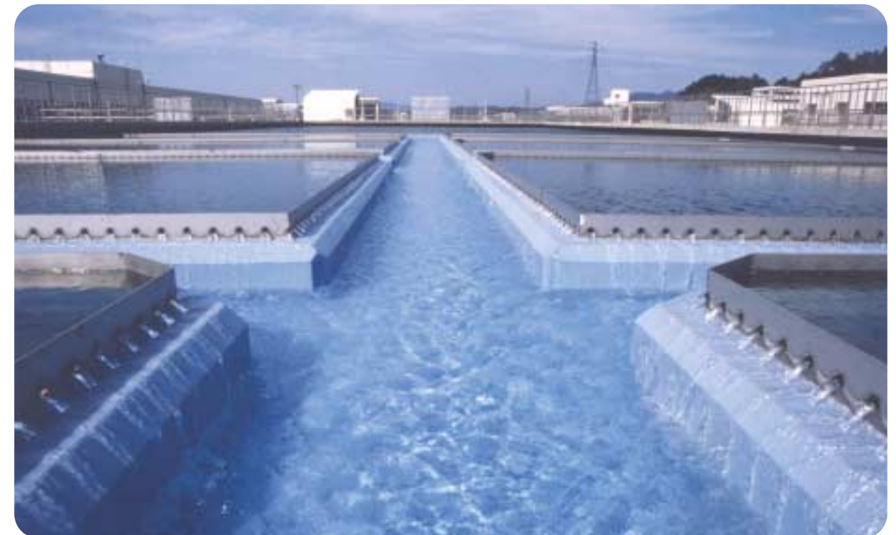
Water purification facility
