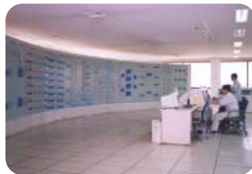
The control center for water purification plant
