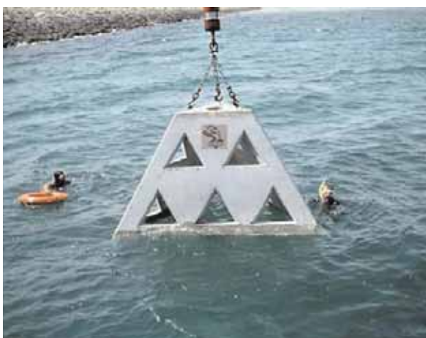
Figure 9: Installation of artificial reef units near the shoreline in Abu Dhabi (Source: Emirates Heritage Club).
