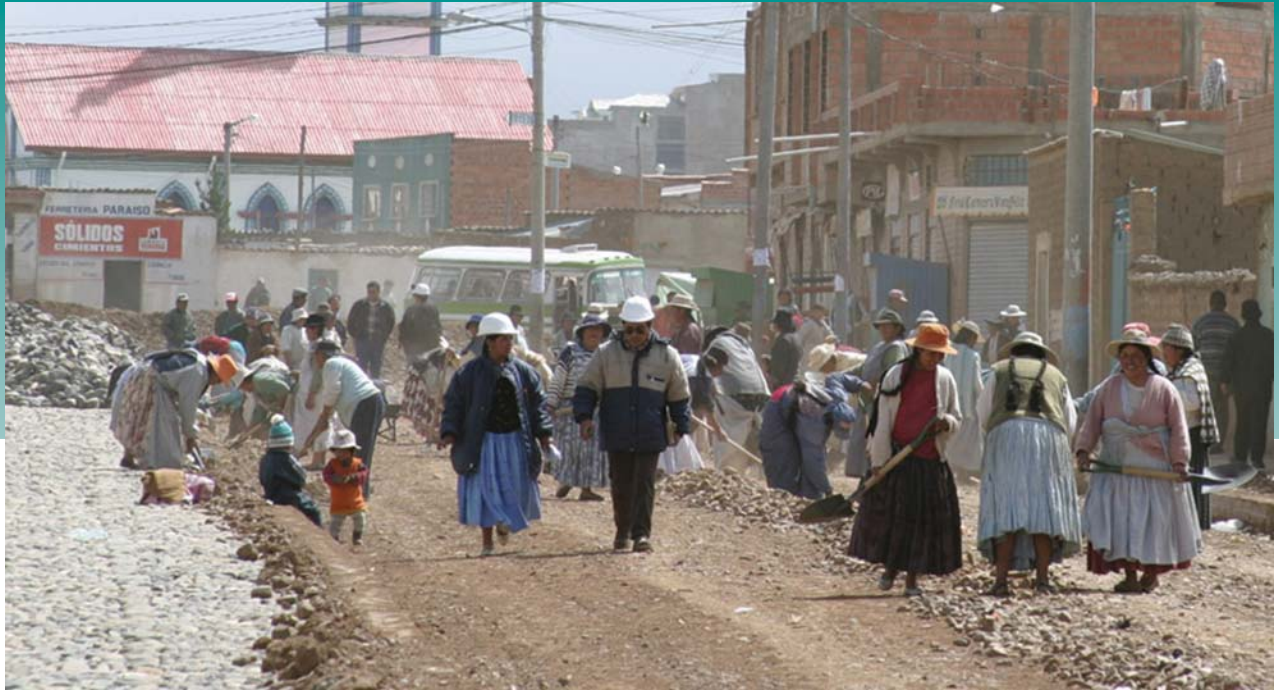
Public infrastructure project (road construction) in El Alto, north of La Paz, Bolivia. Photo credit: USAID.
