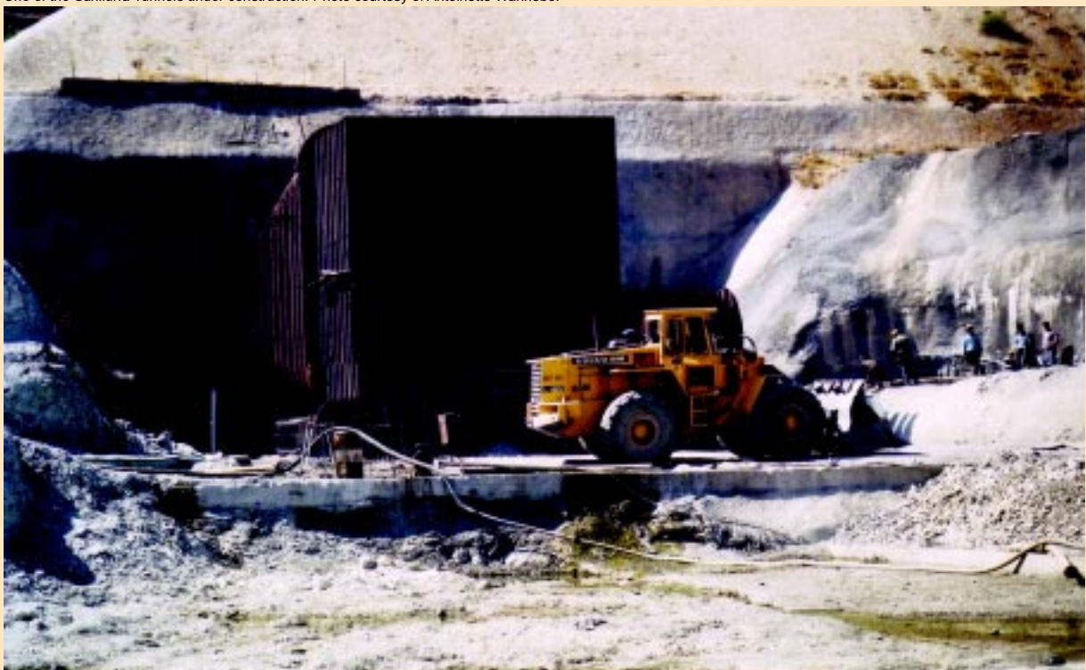
One of the Sanliurfa Tunnels under construction. Photo courtesy of Antoinette Wannebo.
