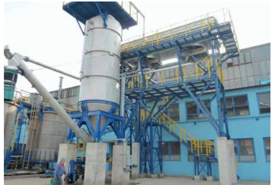
Fig. 19: Secondary lead installation of the company Mach Trade (Slovakia)
